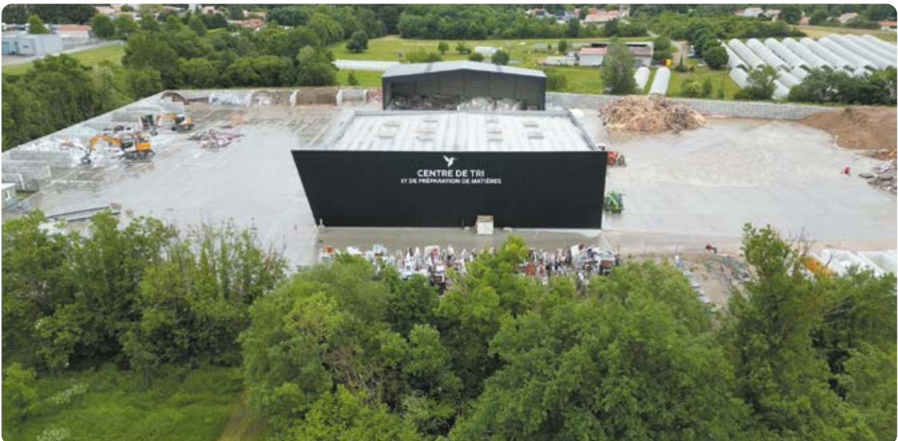
Sorting and material preparation center of EPC Colibri in Le Loroux-Bottereau, France
